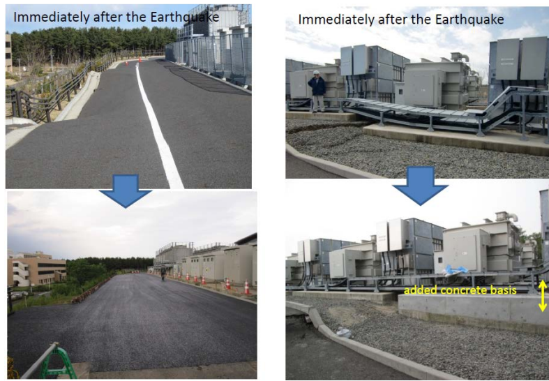
Figure 2. Restoration work of RCS facility. Left: The road was repaved. Right: Tilted capacitors and transformers were straightened after re-leveling the bases.
