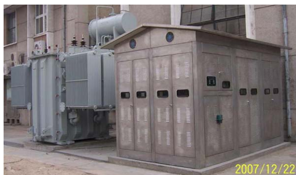
Figure 9 Choke and capacitor bank for White circuit of CSNS magnet power supply.
