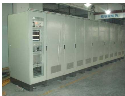
Figure14 The prototype pulse power supply for the injection bump magnet
